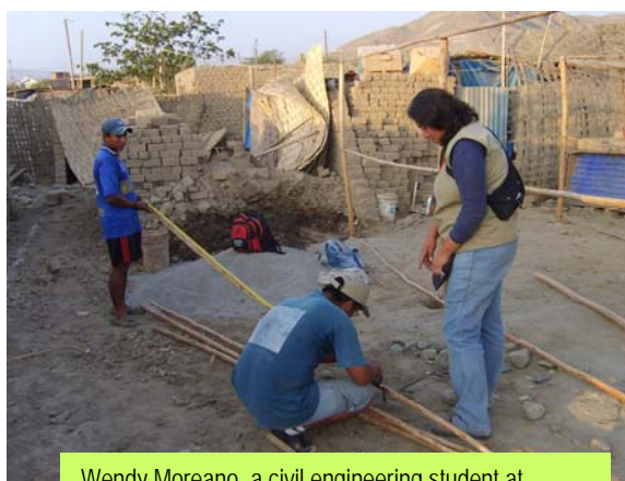
Wendy Moreano, a civil engineering student at Universidad San Luis Gonzaga, provides guidance on how to construct transitional shelters.
