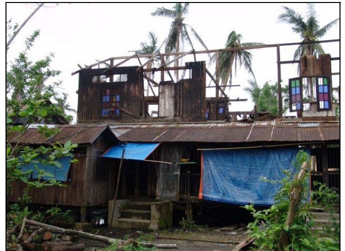
Damaged house in Bogale
